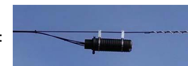
Fiber Coil and Splice Case Mounted on Brackets in Vault:
